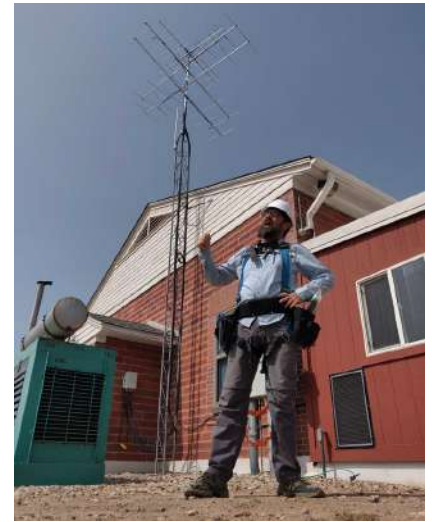
A Motus station is made up of antennas mounted to a new or existing structure, and connected to a receiver and power
