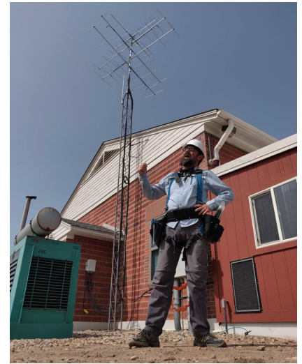
A Motus station is made up of antennas mounted to a new or existing structure, and connected to a receiver and power
