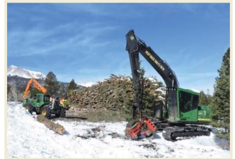
Forest restoration often involves removing trees mechanically with heavy machinery. Material removed from restoration projects becomes lumber, firewood, mulch and more. Photo: T. Woodward.
